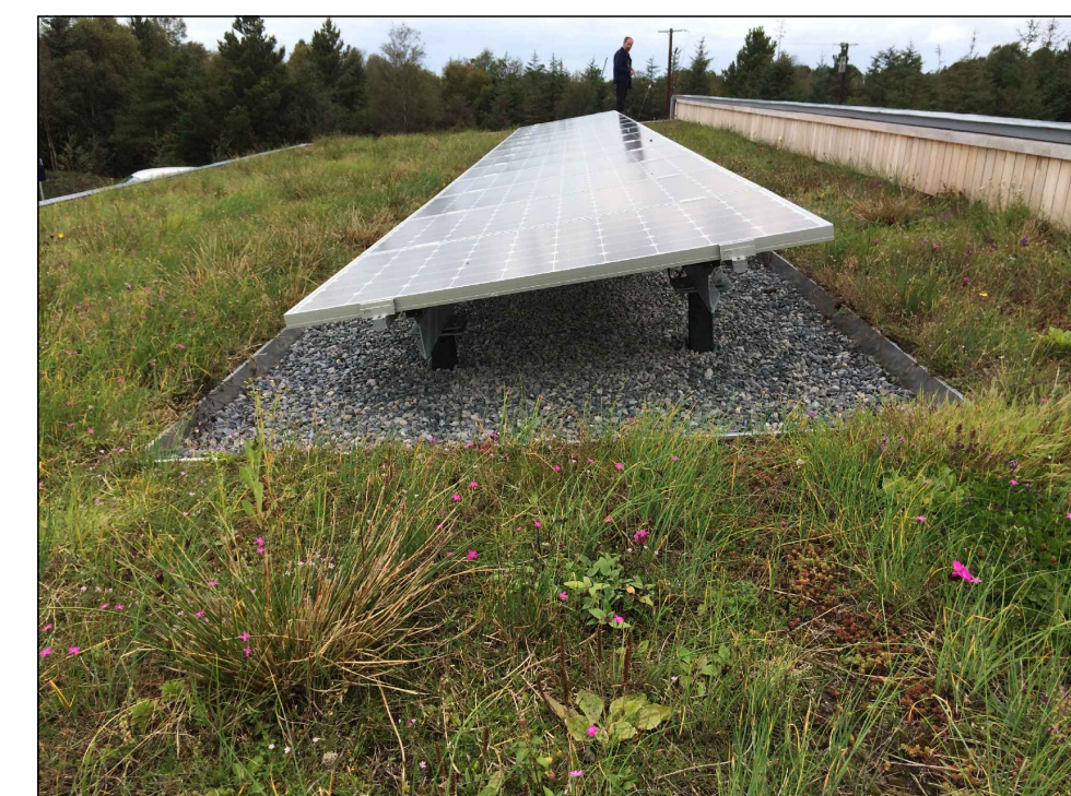
PV PANEL ON GREEN ROOF
